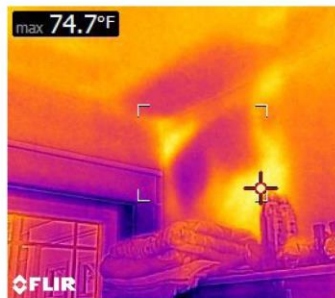
Missing Insulation – Summer Day E6 with MSX
